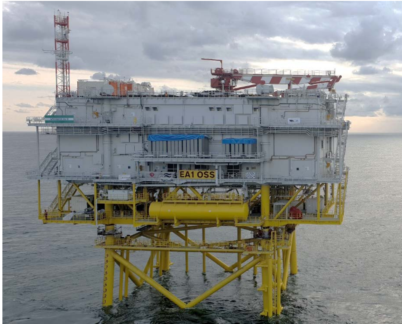
Plate 3:4 Offshore Electrical Platform
