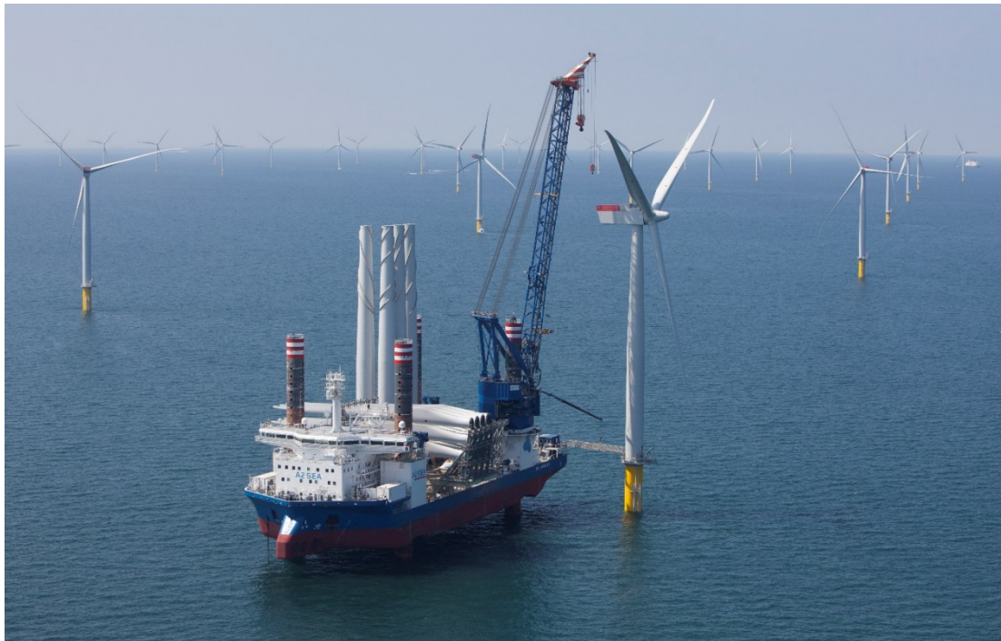
Plate 3:5 Wind Turbine under Construction (photo taken from West of Duddon Sands offshore windfarm)
